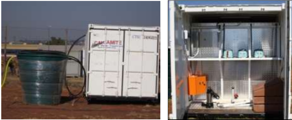
Fig 19: Containerised waste water treatment plant
