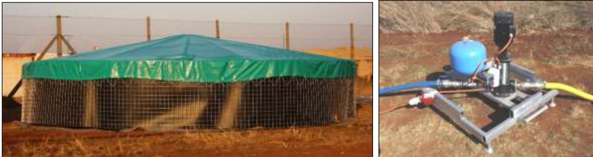
Fig 17: Mesh tank for water storage (left) and booster pump station (right)
