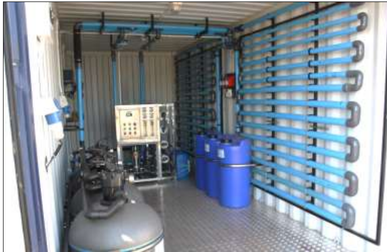
Fig 16: The 50-man Water Purification Plant
